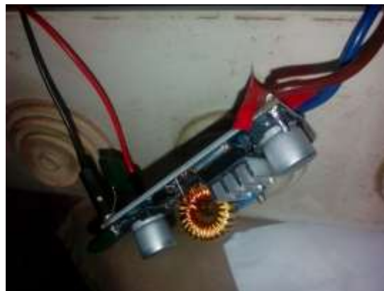
Figure 6: Regulator between solar controller and circuit boards
