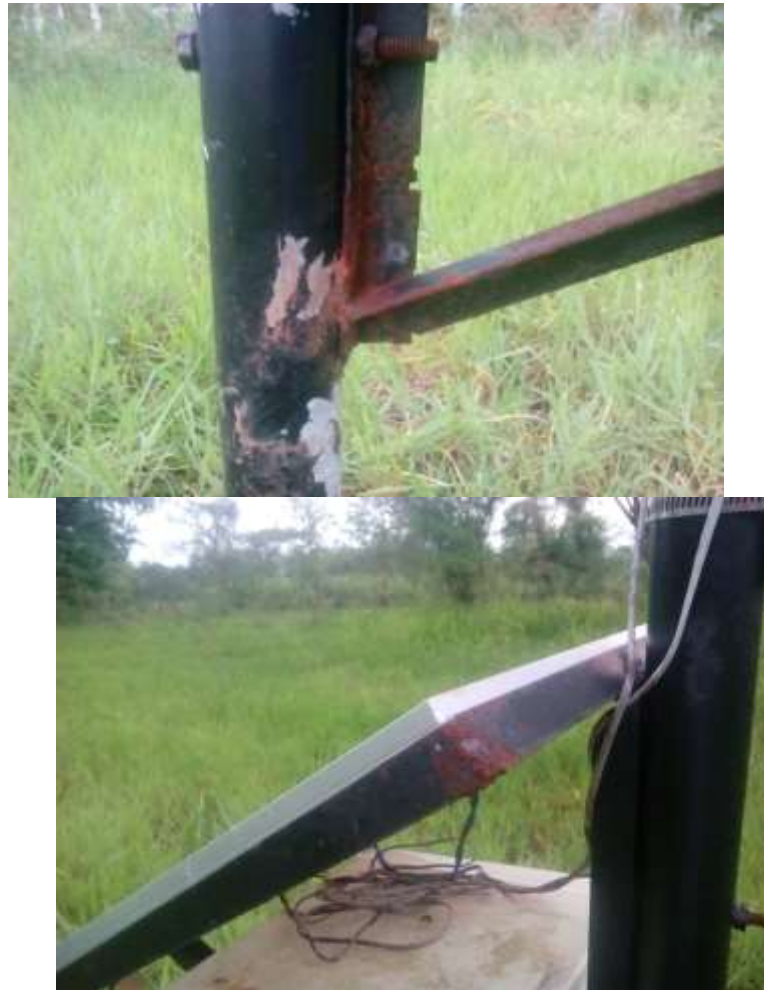
Figure 10: Signs of aging of the pole structure: rusting.
