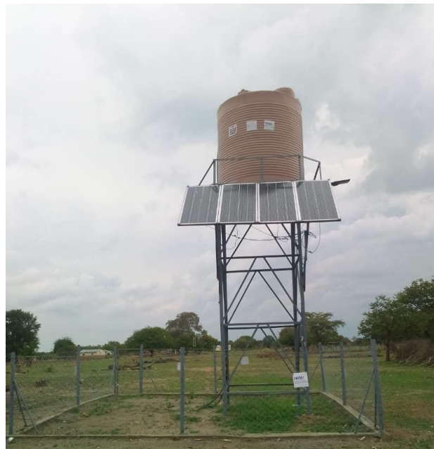
Figure 9: Solar-powered borehole infrastructure implemented for Hanzila village as a multi-purpose water infrastructure
