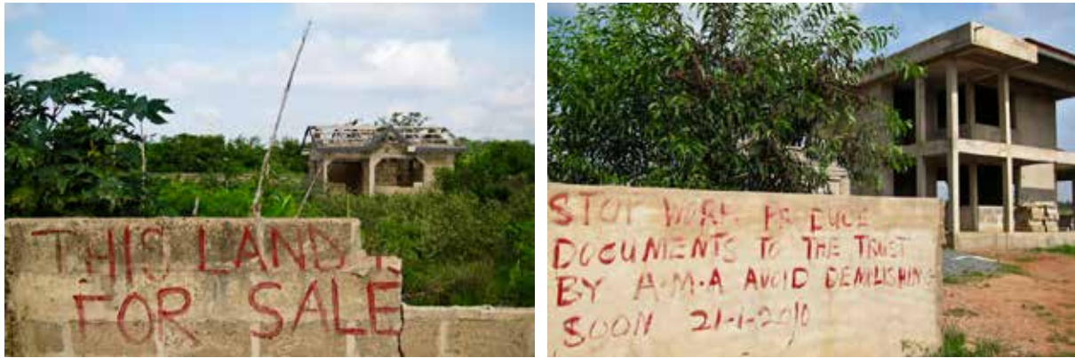
FIGURE 13.2. Demolition threats on unfinished structures peppering the La site (photos courtesy A. Allen).
