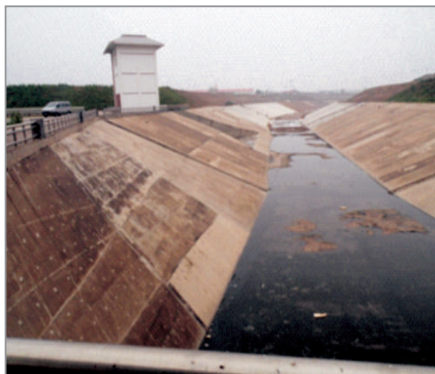
Figure 1 A picture of the middle route (near Shijianhuang) of the three canals of South-to-North Inter-basin water transfer project
