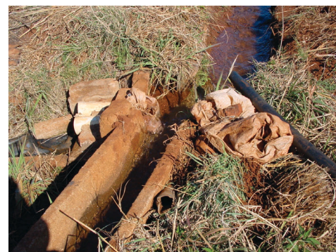
A disintegrating irrigation canal in a rural village in Hereford South Africa shows there is a need for improving rural infrastructure to help the poor.
