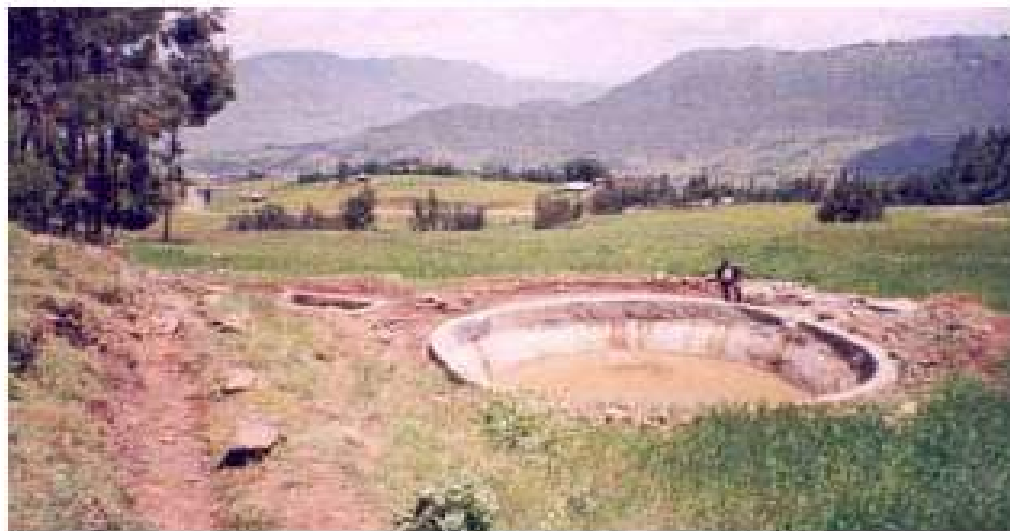
Leaking from outside in: Hemispherical tank built on a slope in Dessie Zuria with groundwater seeping through the walls into the tank (photo H. Rāmi, UN-OCHA, Oct.
