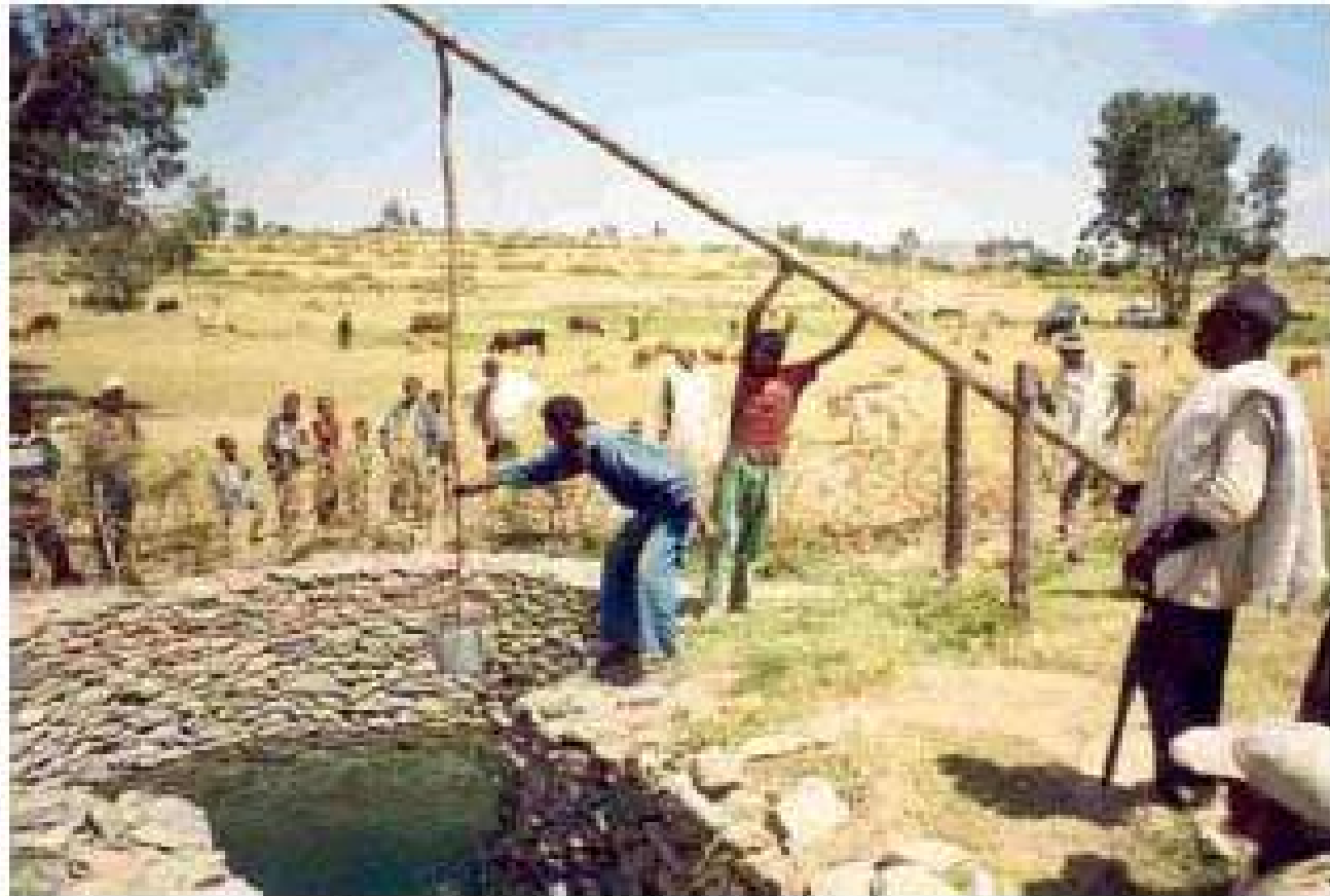
Groundwater discovered while excavating ponds:
