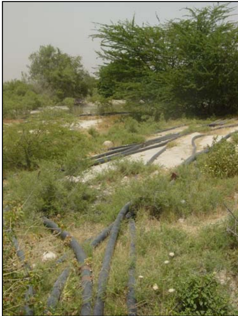
Picture 1: Privates pipes running in the southern part of the valley
