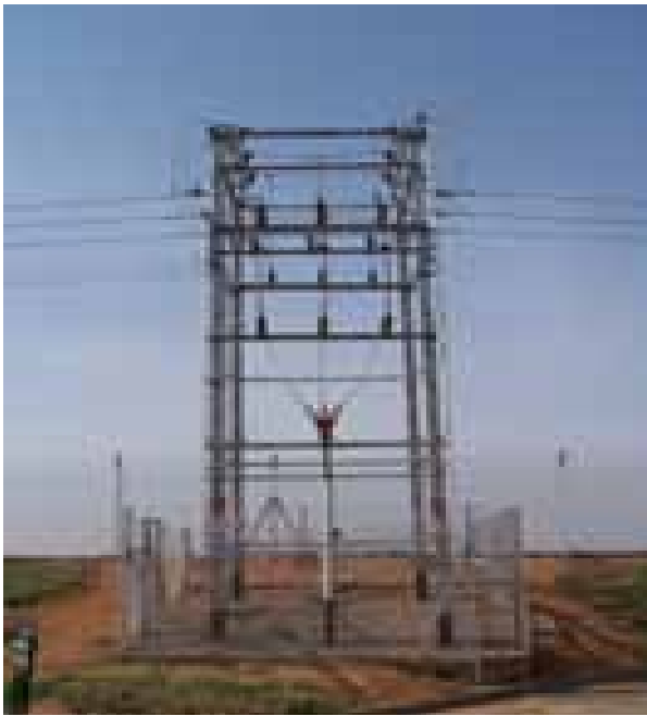
In Gujarat, separating the power cables carrying electricity to farmers from those supplying other rural users, such as domestic households and industries, had positive impacts much greater than anticipated. Photo Credit: Terry Clayton, IWMI.
