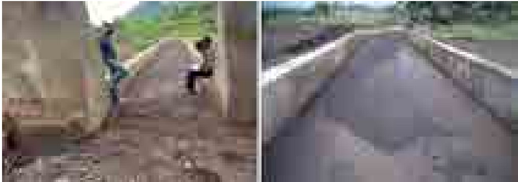
Figure 9.4. Sedimentation at the Fokisa offtake and canal systems
