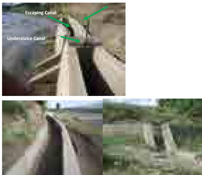
Figure 8.5. Golina spate irrigation project, headwork and canal structures.
