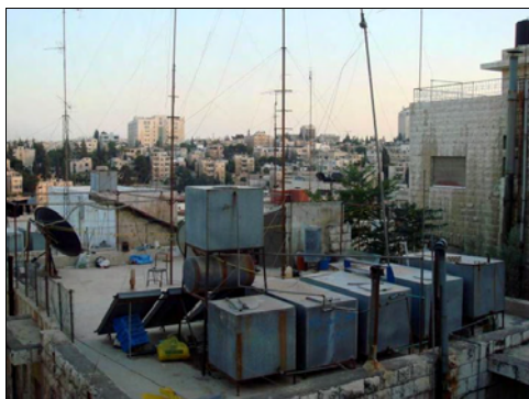
Figure 5-41. Roof top water cisterns in Amman (Venot, 2007)
