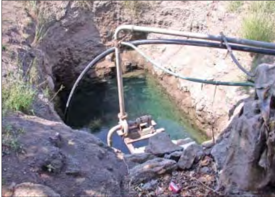
Figure 22. Electric and diesel pump is used in the same well.
