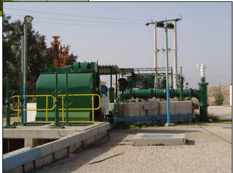
Picture 3. A pumping station within the Jordan Valley
